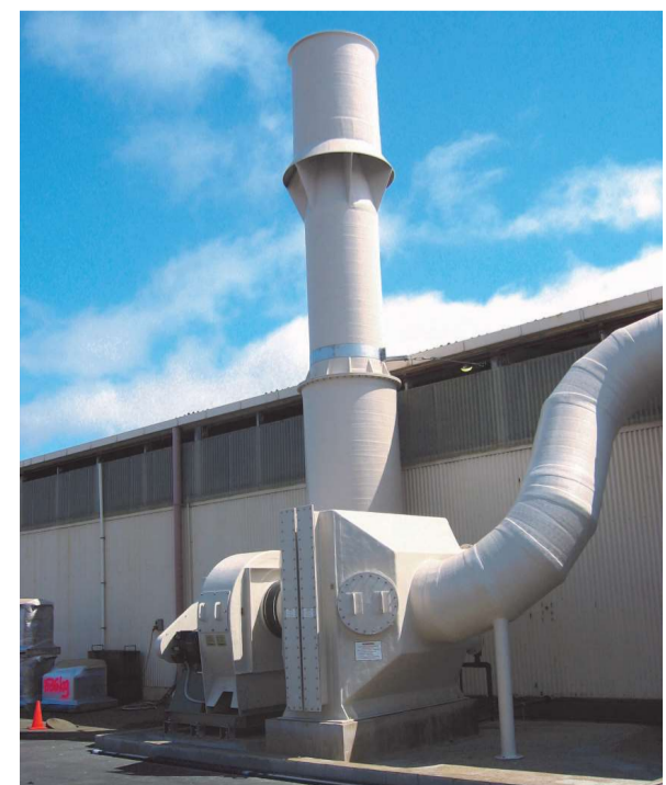
Service life # 1: Armatec designed, manufactured and installed the air pollution control systems to fit a client's site.
