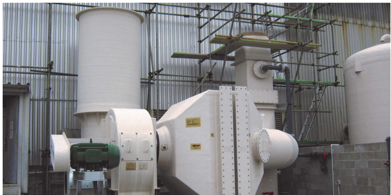
Armatec repurchased, repurposed and modified to reuse the scrubbing system at a customer site.
